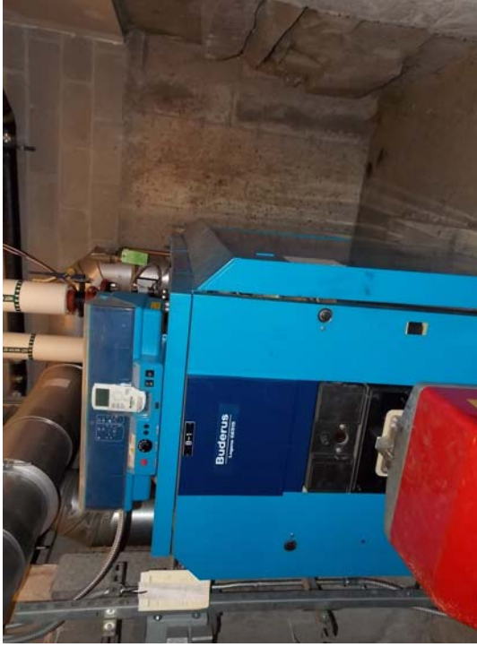
This is the new oil-fired boiler.
