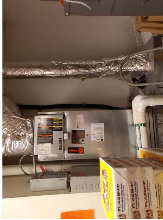
One of the air handlers.
